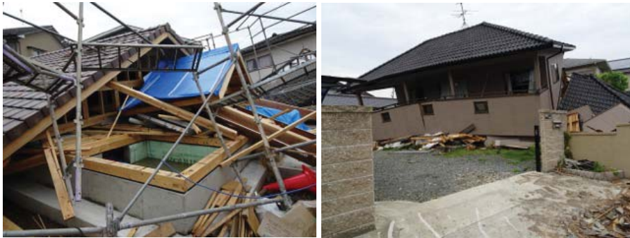
Photo. Damage of the dwellings caused by the Kumamoto earthquake in Mashiki Town
