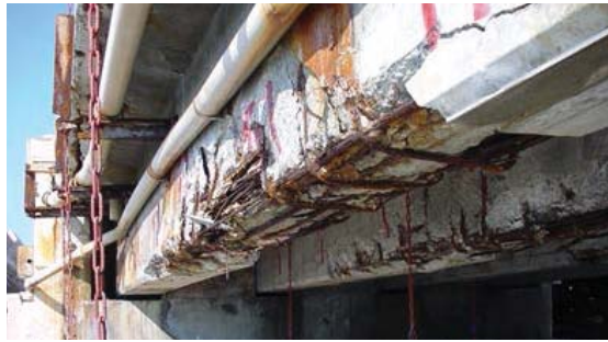
Fig.1 A concrete structure damaged by chloride attack
