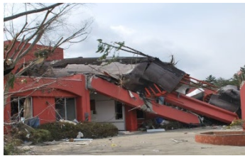
Fig.1 Elderly facility broken by the tsunami of March 11, 2011
