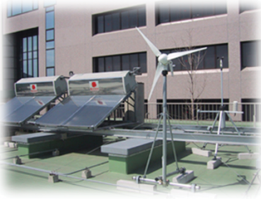
Renewable energy system
